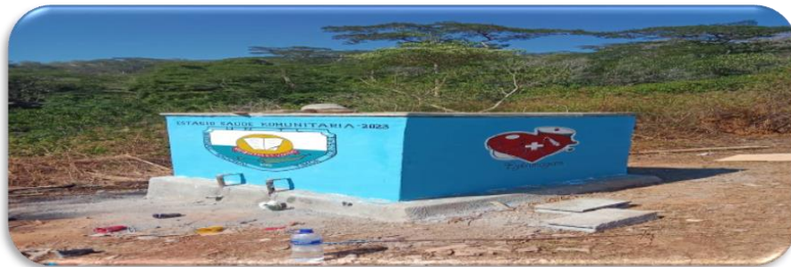
Figure 6. Potable water tank in Rae-Udo
